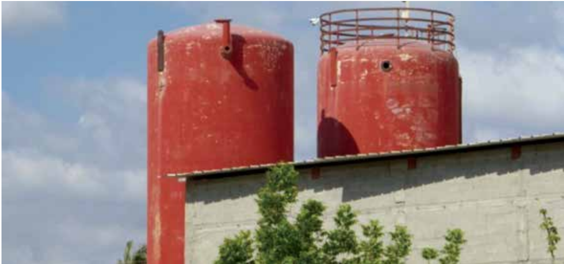
Geshuri & Sons, Tulkarem: is this a 'Bhopal' waiting to happen?
